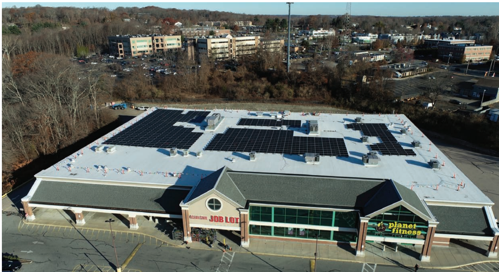
RAISE THE ROOF: A Rhode Island based solar energy company has installed 750 solar panels on the roof of Ocean State Job Lot's store at 1493 Hartford Ave., in Johnston. (Submitted photo)
